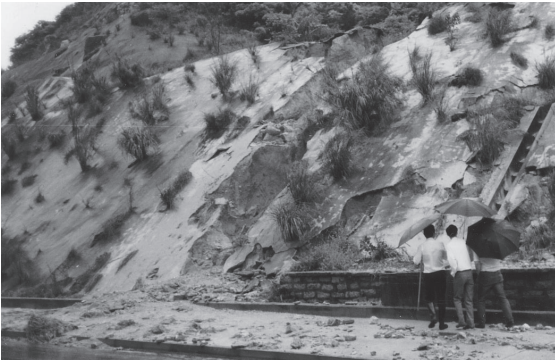
Figure 4. General view of failure - case 1
