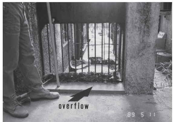
Figure 7. Accumulated dead leaves as evidence of overflow - case 2
